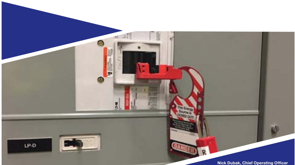
Nick Dubak, Chief Operating Officer Dubak Electrical Group
